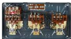
Interior View of MK2 SASD
