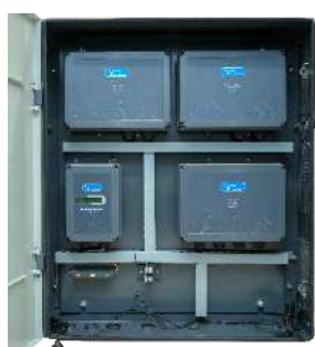
Interior View of xMasm10 - Wired Solution
