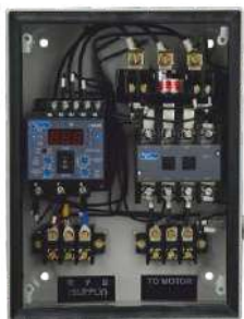
Interior View of MD Starter+ DOL Starter
